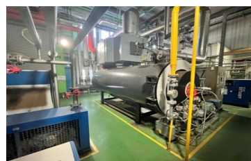
Low-NOx Boiler (3 tons)
