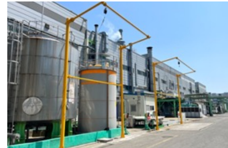
Oil Tank Safety Structures
