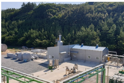
Wastewater Treatment Facilities
