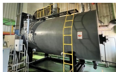
Low-NOx Boiler (10 tons)
